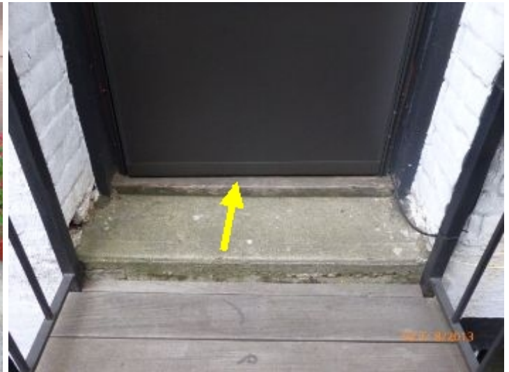
Exposed wood saddle at rear entrance door
