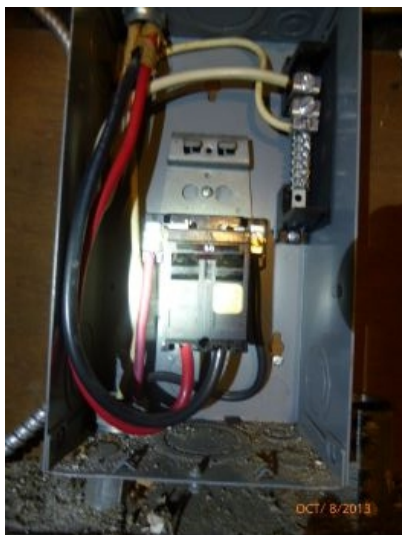
Electrical Main Service Panel(s)
