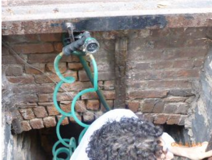
Deteriorated mortar at ventilation shafts
