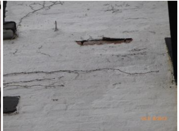
Patch of missing cement cladding
