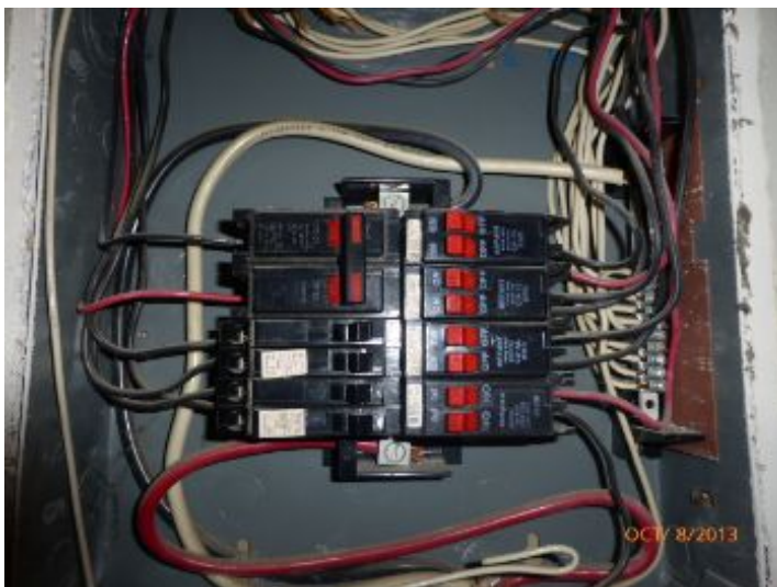
Electrical Main Service Panel(s)
